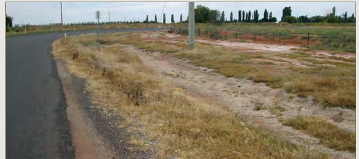
Plate 15 Soil compaction for road construction impedes groundwater movement and may restrict surface water drainage. The result is waterlogging and salt concentration beside the road. Source: Southern Salt Action Team (2003)
