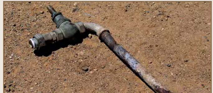
Plate 32 Galvanised pipes corrode prematurely. Source: Southern Salt Action Team (2004)
