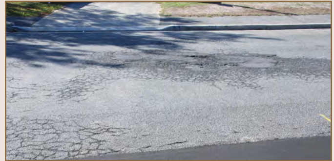
Plate 30 Damaged road surfaces in the greater Launceston area due to salinity. Source: Armstrong, D. (2007)
