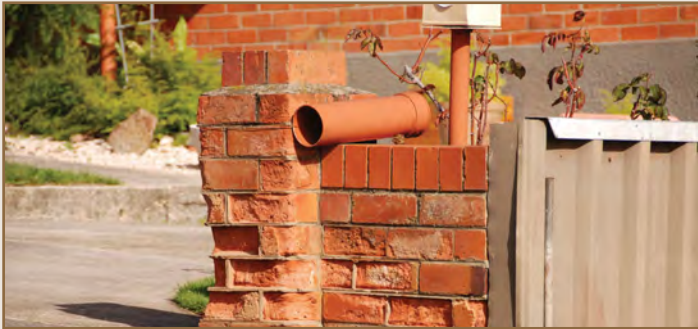
Plate 29 Salt damage to bricks and mortar in northern Tasmania. Source: Armstrong, D. (2007)
