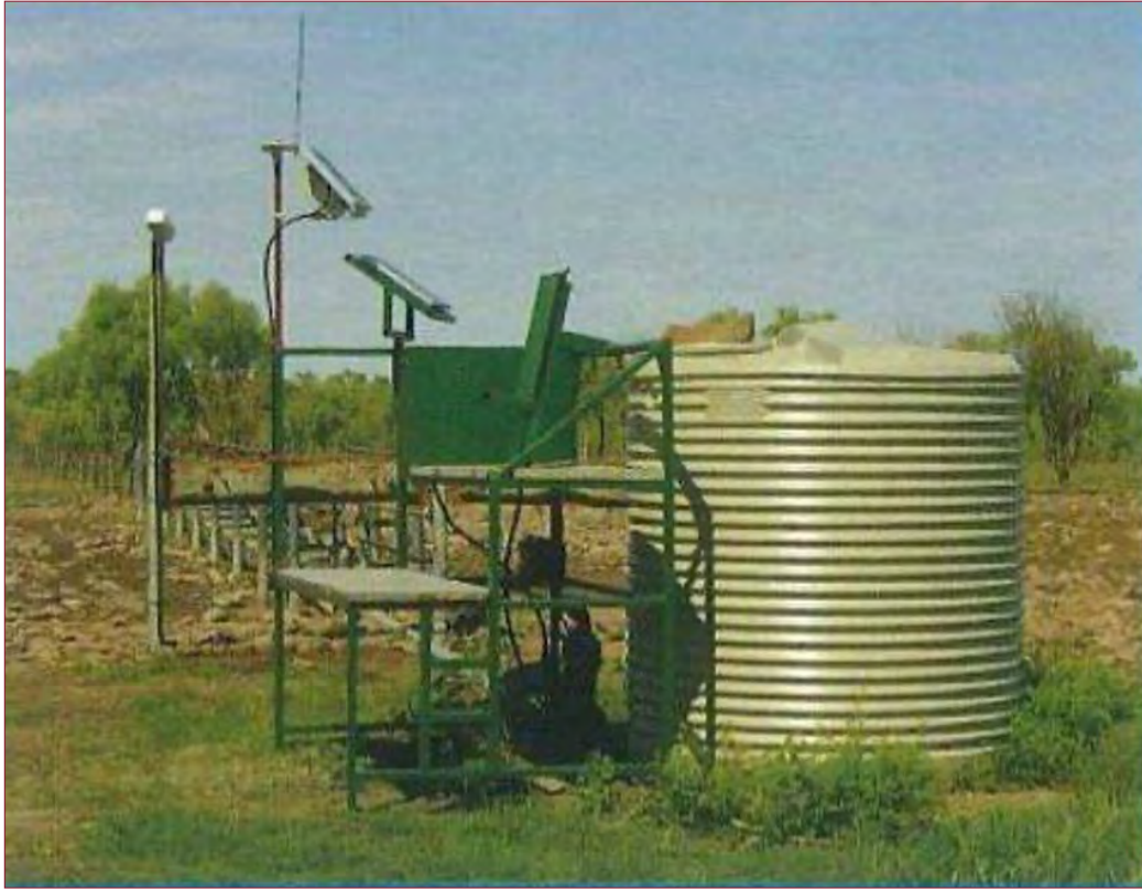
Figure 14: Tank and trough formation with solar panels and telemetry
