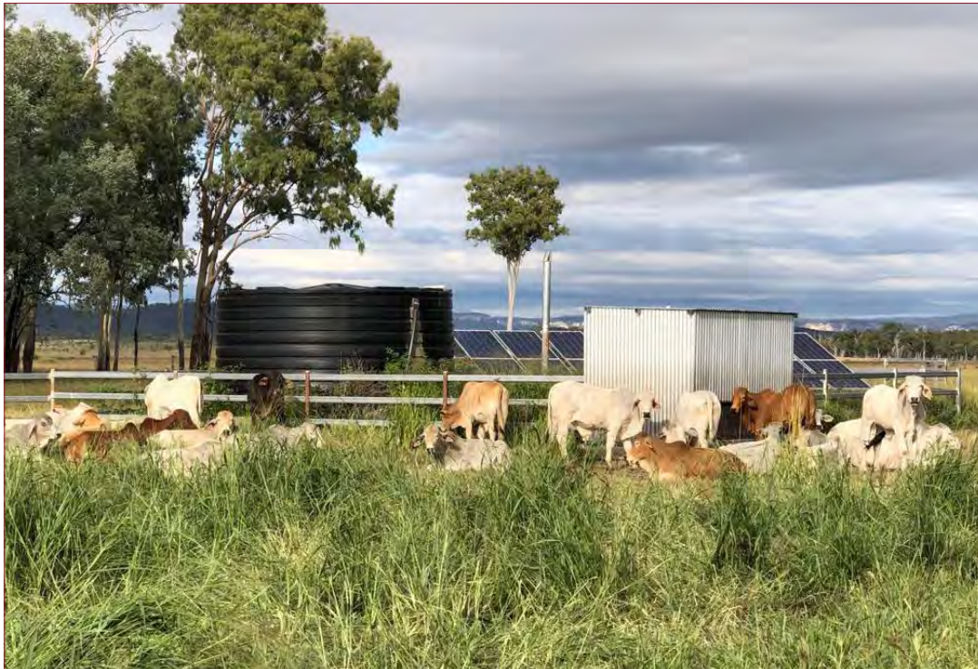
Figure 12: Fenced off solar array, bore house, and tank near Carnarvon Gorge, Queensland
