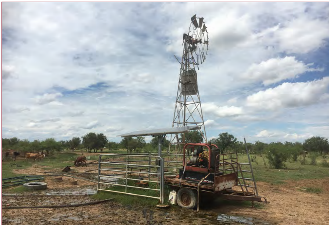
Figure 11: Example of a diesel pump at a bore as a temporary measure
