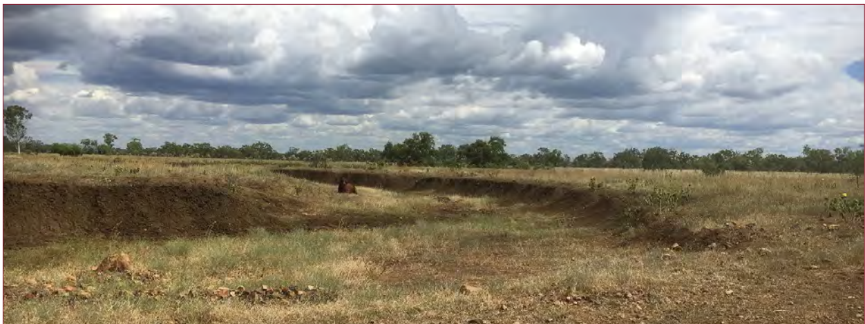
Figure 26: Poorly-constructed flat-bottom drain, now stabilised, Kimberley Region, WA
