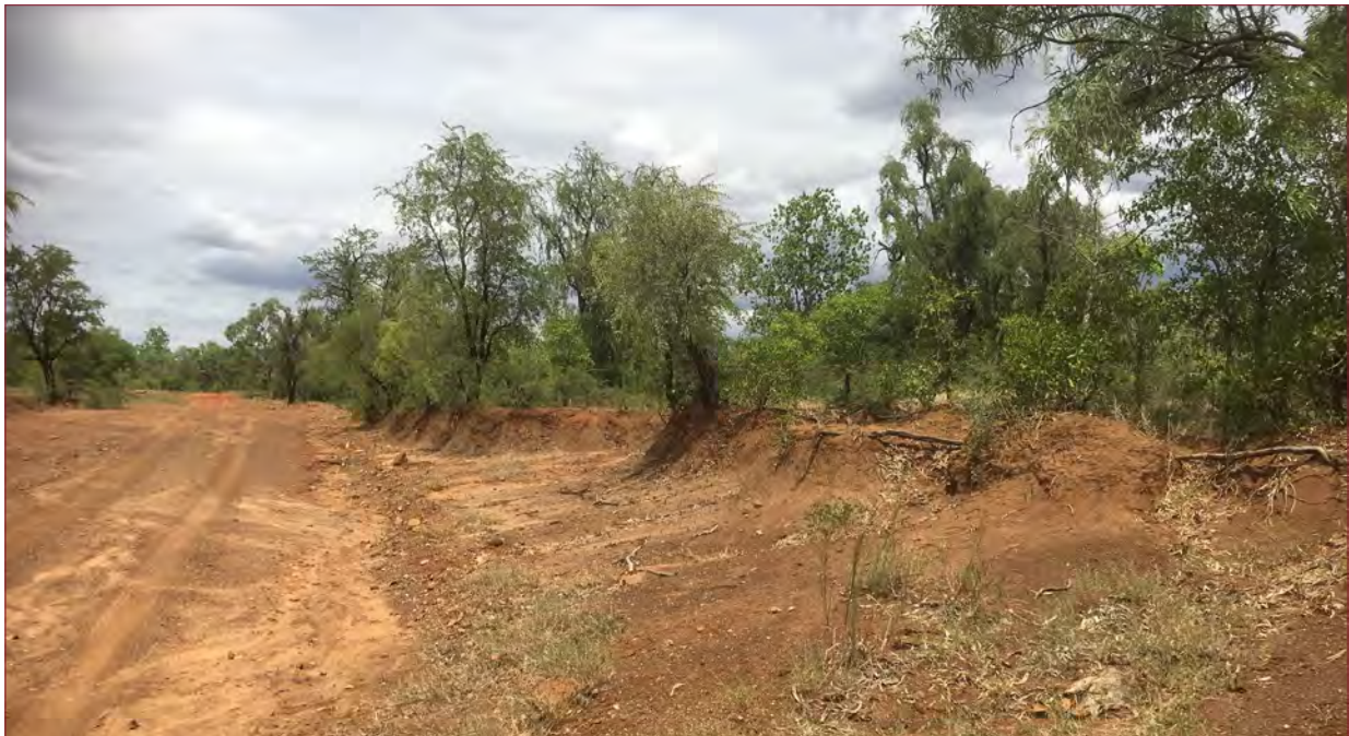
Figure 19: Example of poorly constructed road in hilly terrain, Kimberley Region, WA
