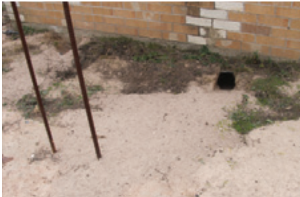
Pic. 11 : Rabbit hole under building.
