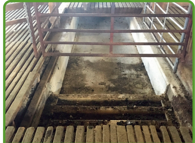
Hidden solution: Permanent concrete footbath under slats in shearing shed. When the footbath is not in use, the grating sits back over the footbath allowing for normal use of the shed.
